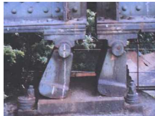
Fonte: BRIDGE INSPECTION MANUAL – NY'S DOT
