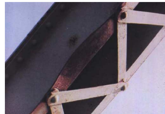
Fonte: BRIDGE INSPECTION MANUAL – NY'S DOT
