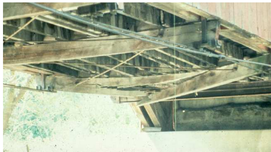
Fonte: BRIDGE INSPECTION MANUAL – NY'S DOT
