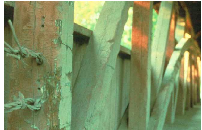
Fonte: BRIDGE INSPECTION MANUAL – NY'S DOT
