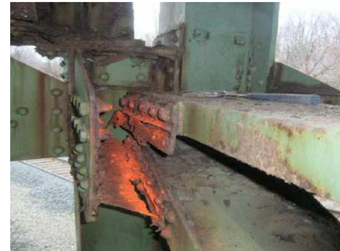
Fonte: BRIDGE INSPECTION MANUAL – NY'S DOT
